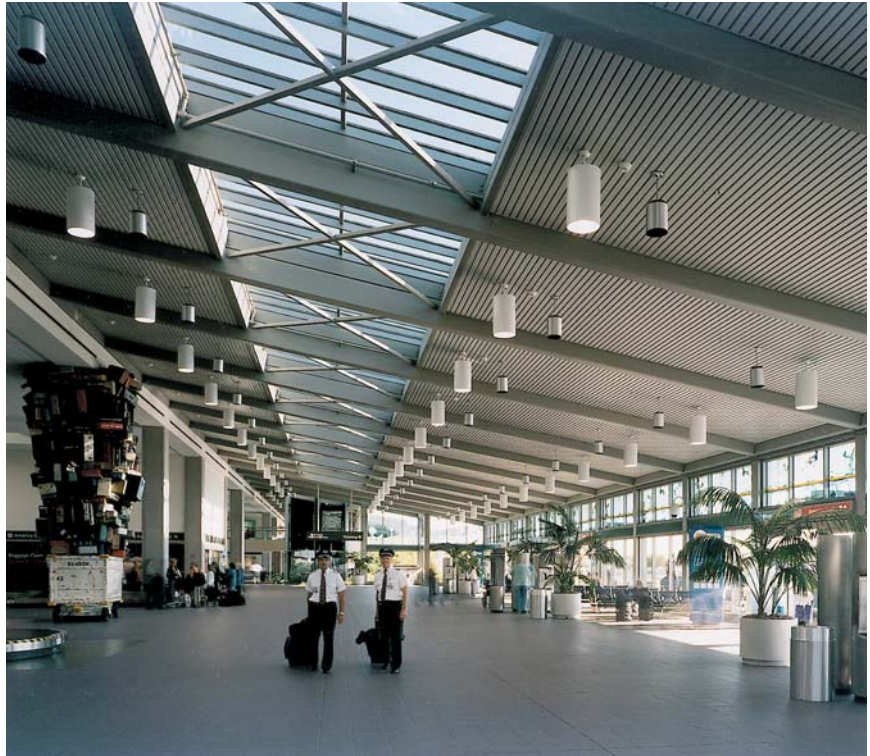
Sacramento International Airport, Terminal A, Sacramento, CA Architect: Dreyfuss & Blackford, Photo: Cathy Kelly Architectural Photography, A/D FIREFILM® II on beams
